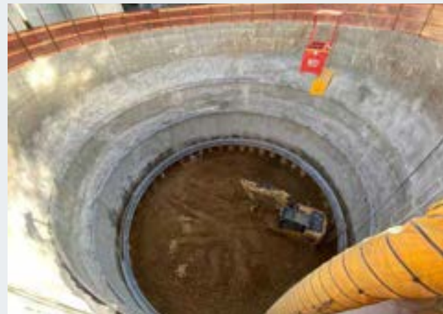
Paschiera Water System - Duplication of the Aqueduct | ACEA , Tivoli, Italy Water System Management
