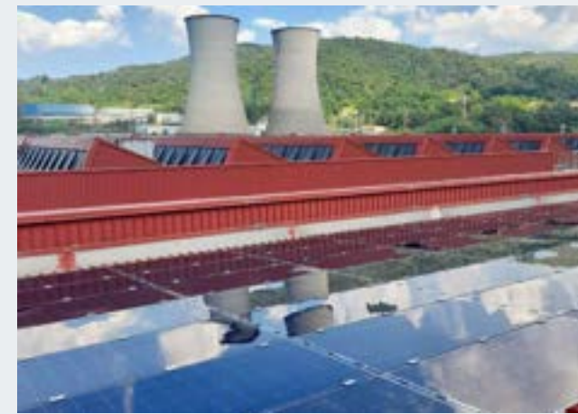
Photovoltaic System | Enel Italia Lardello, Italy
