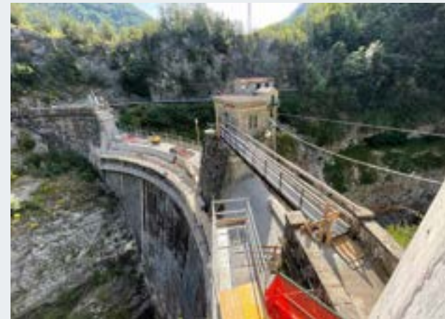
Gangheri Dam | Enel Green Power Italia Lucca, Italy Commissioning Services
