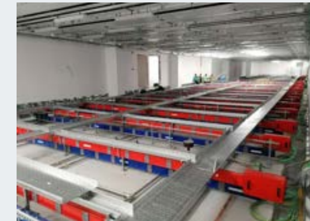
Data Center | NOOVLE Rozzano, Italy Works Supervision
