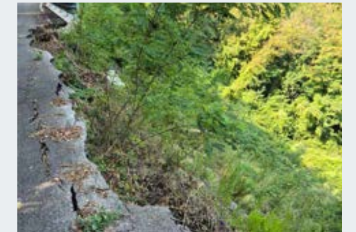
Castel San Pietro | CONSAP Bologna, Italy Landslide Emergency
